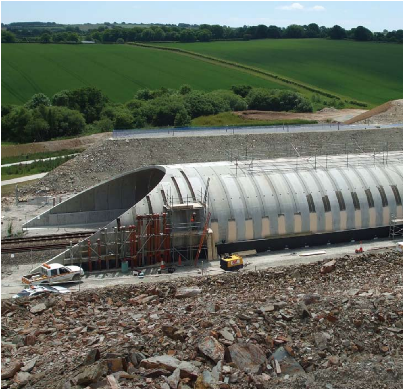
BEBO pre-cast concrete arch for the A38 Dobwalls Bypass over the London to Penzance rail line
