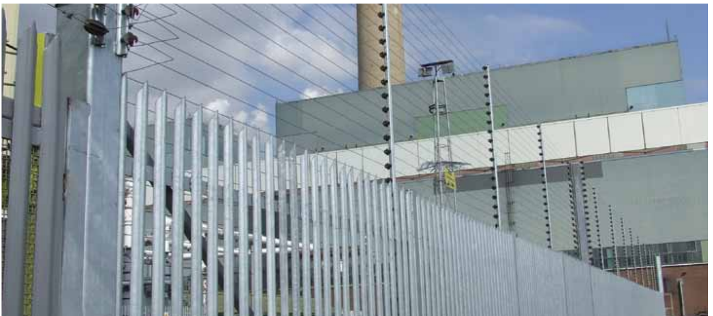
Barkers StronGuard security fencing installed complete with a full length electric fence, protecting a CNI listed sub-station.
