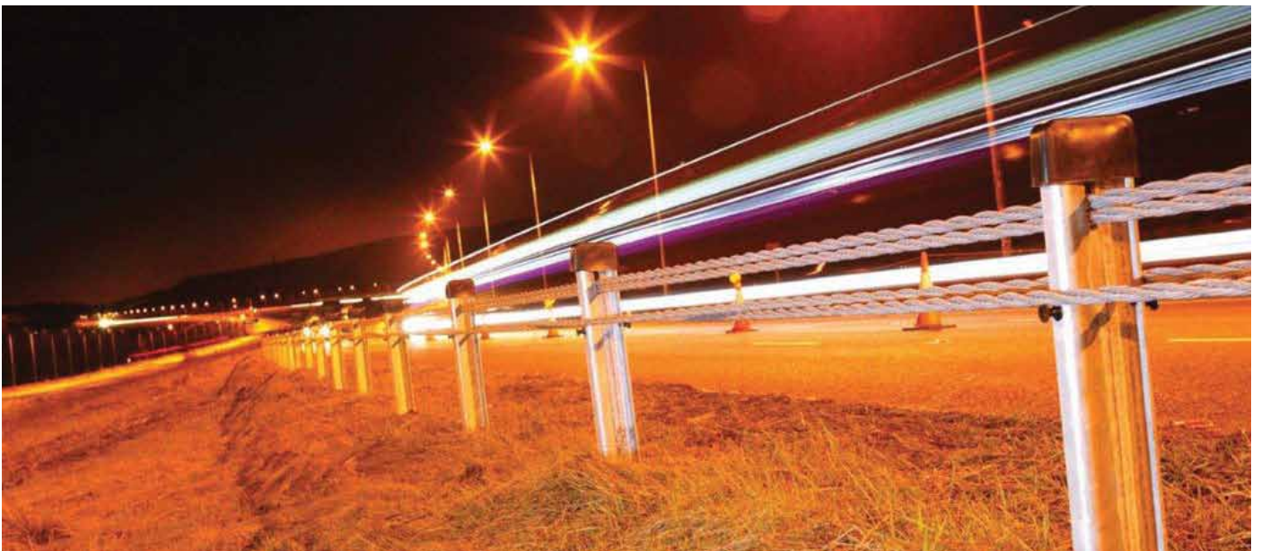
An installation of our Brifen wire rope restraining system.
