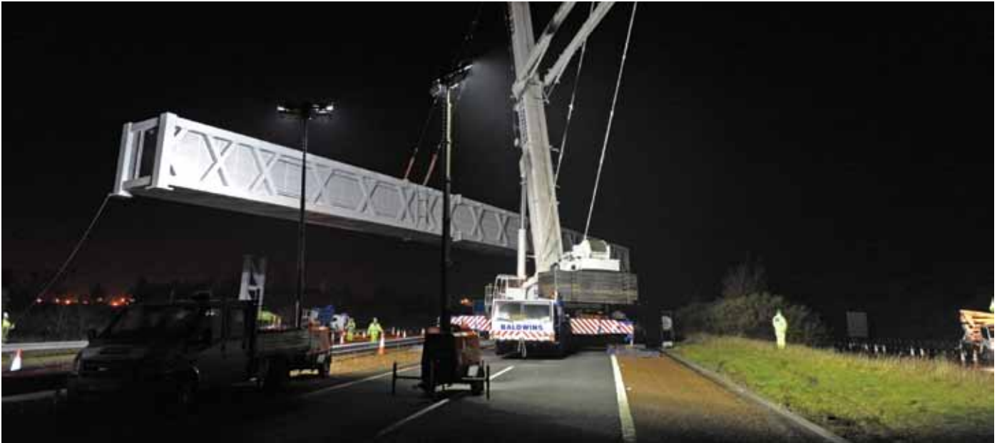
Access Designs' newly designed and manufactured gantry being installed close to junction 2a on the M90 in Scotland.
