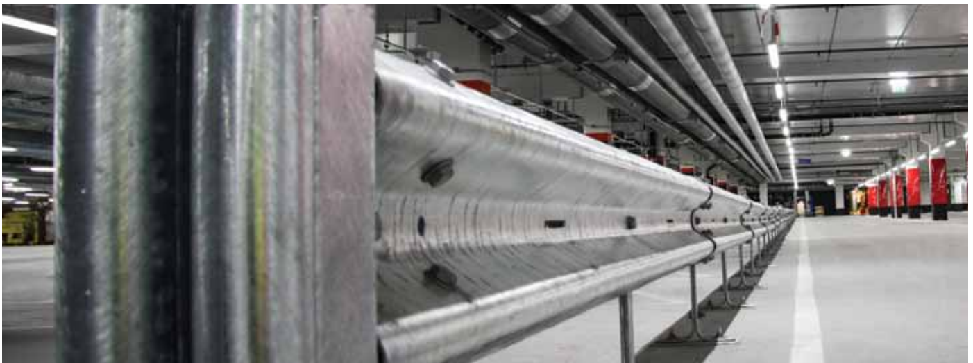
700m of Berry parking barrier at the Tele2 arena, the new multi-purpose stadium in Stockholm.
