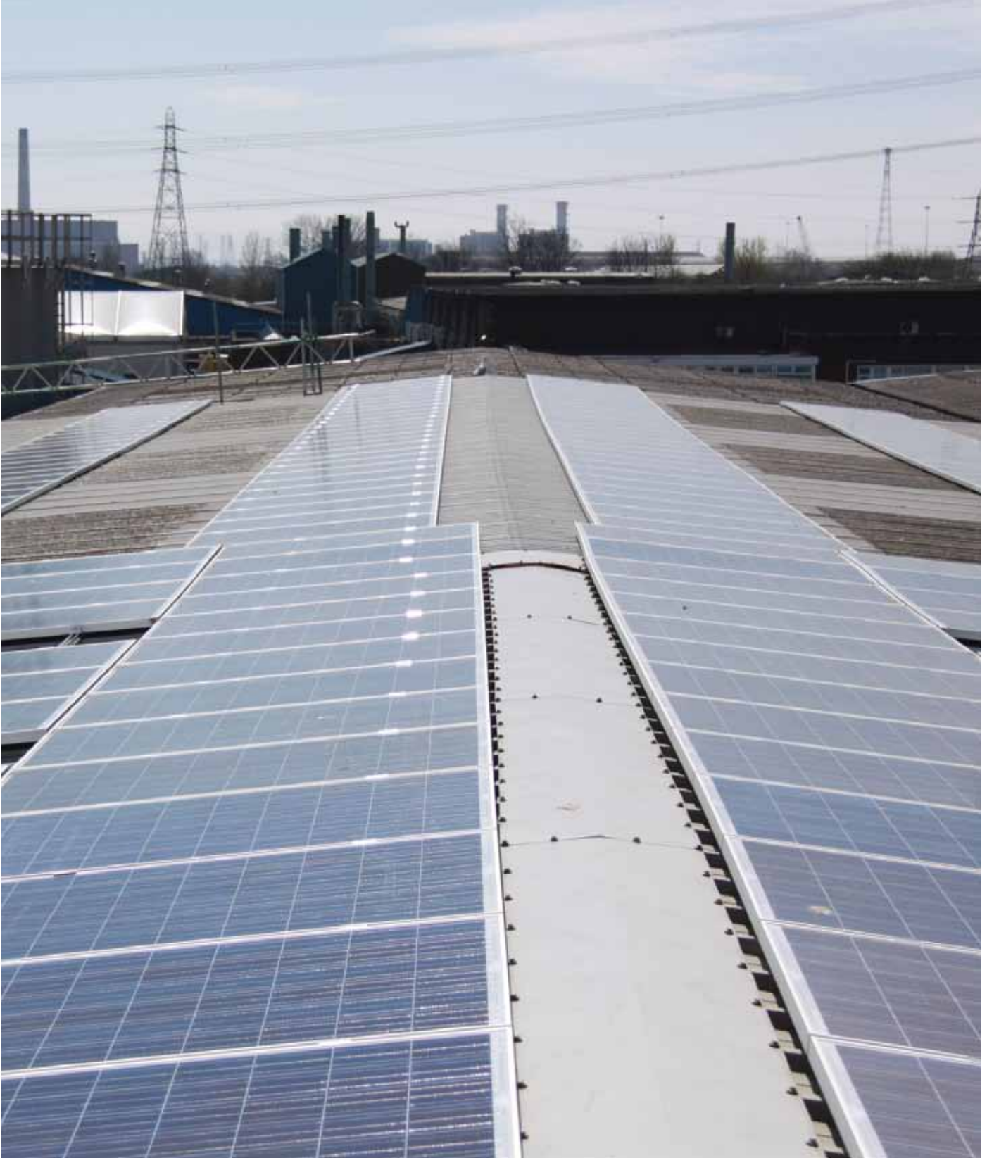
Solar panel installation at our Asset Weholite factory, Newport, South Wales, referred to on page 29.
