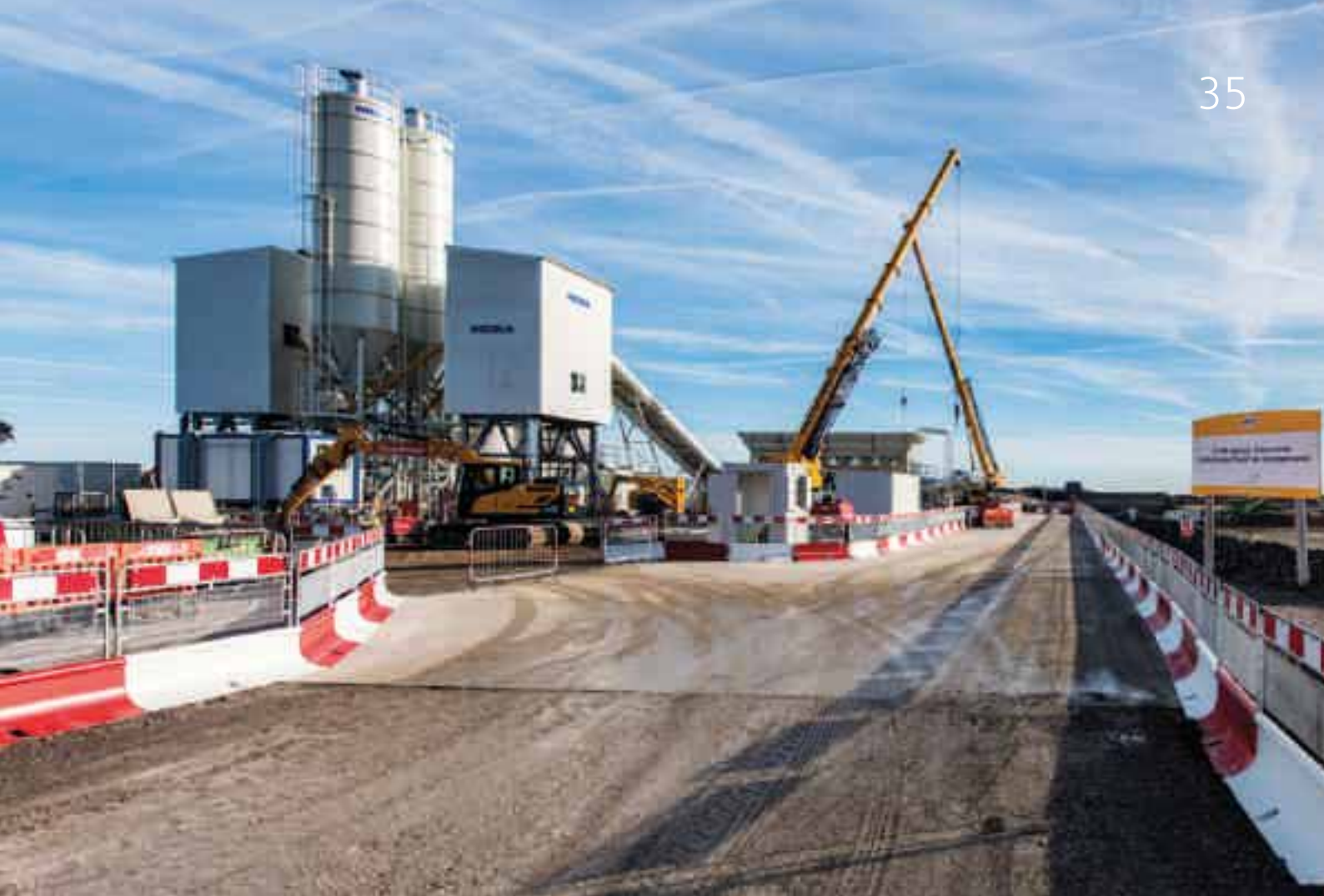
M.A.S.S. Visirail guard supplied by Asset VRS at Hinkley Point C nuclear power station, Somerset.
