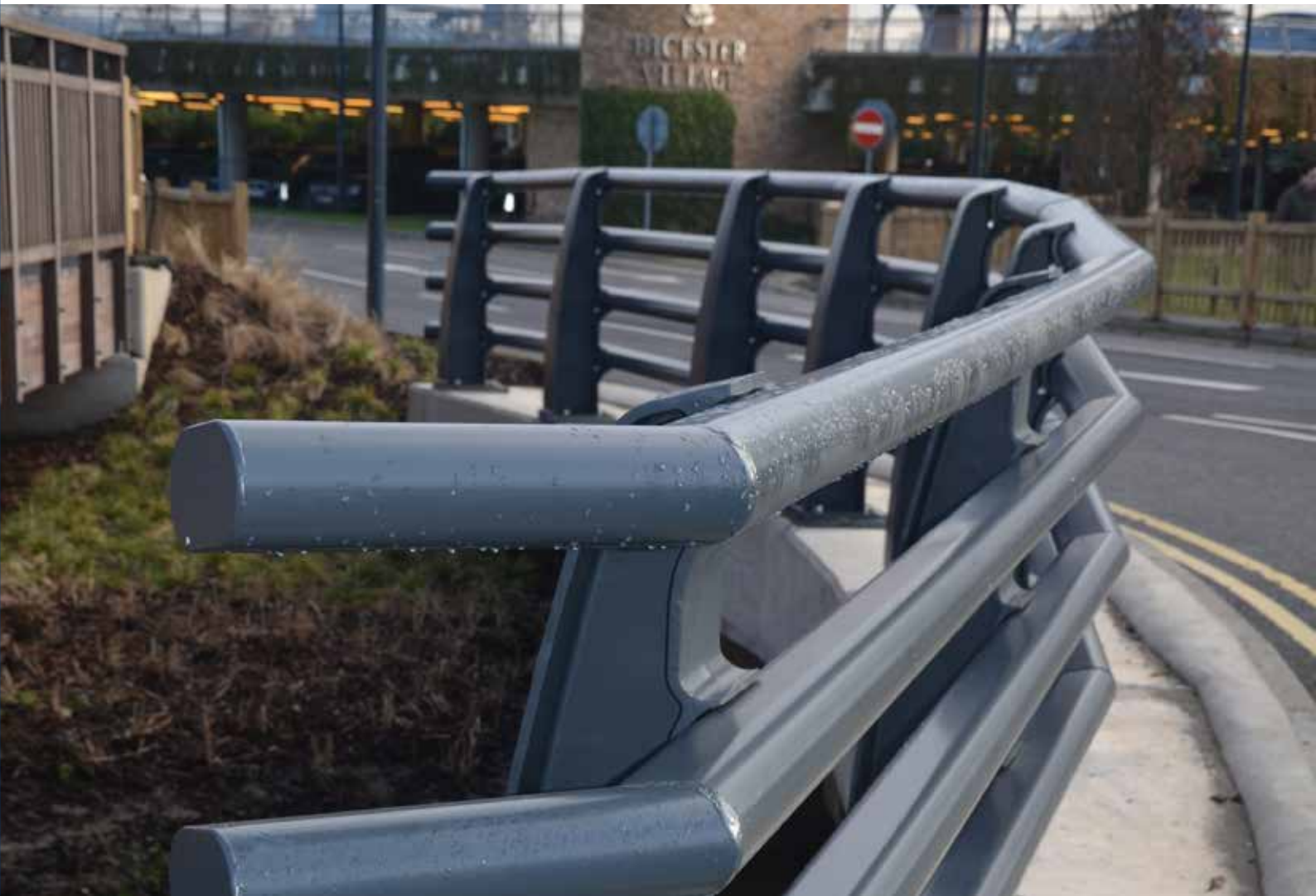
Bottom: VGAH 2000 Aluminium H2 Parapet, by Varley & Gulliver Ltd, installed at Bicester Village. The first time H2 Aluminium parapet has been used in the UK.
