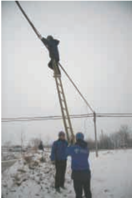
China Telecom staff were striving to recover the telecommunications cabling damaged by the snowstorm
