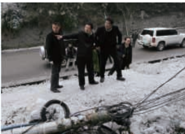
Chairman Wang Xiaochu (Left 2) inspected the damages to the telecommunications facilities brought by the snowstorm in Guizhou Province and led the recovery works
