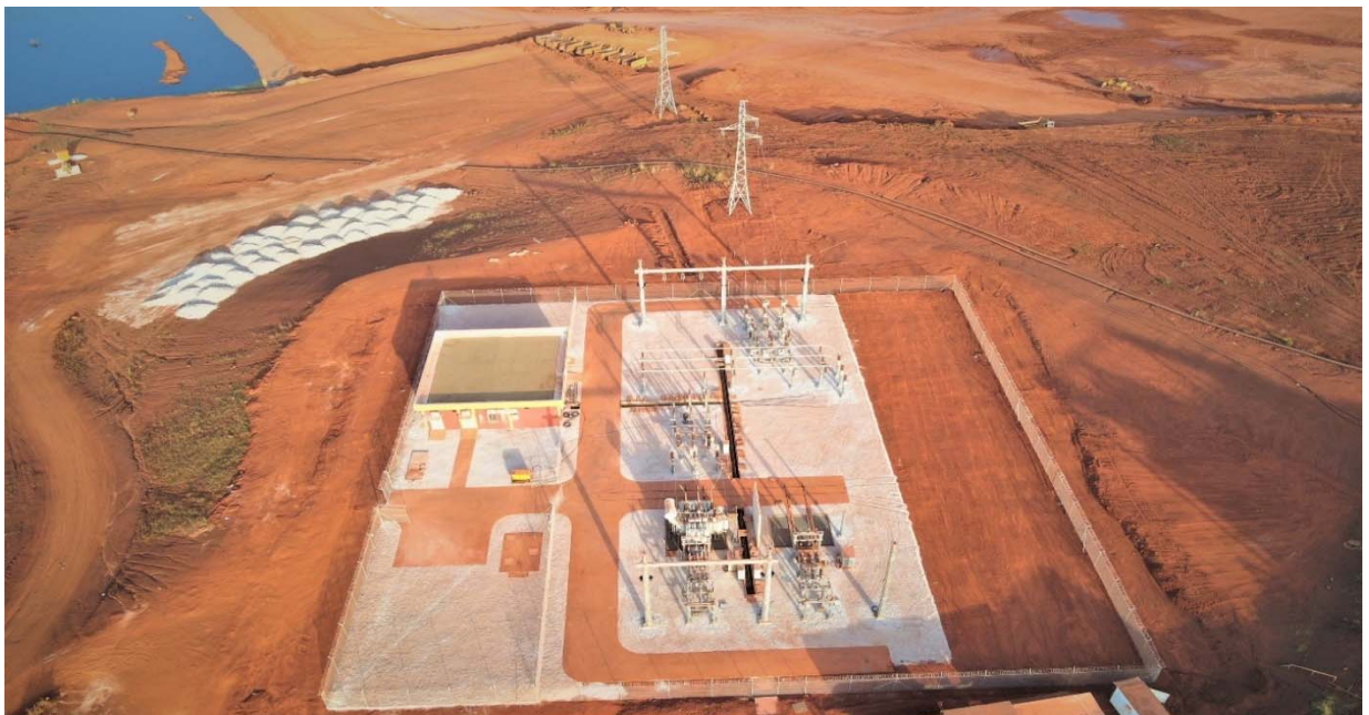
Figure 8: Abujar 90kV substation
