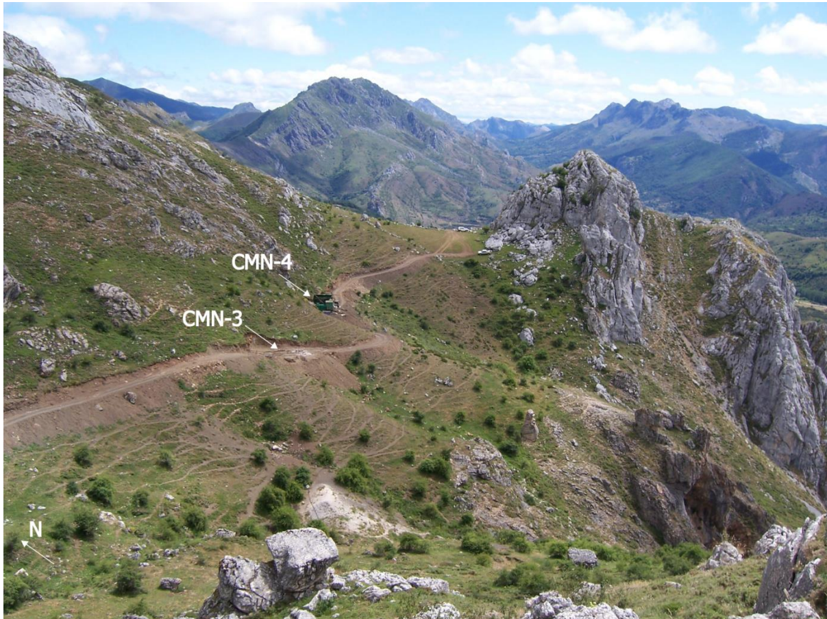
Figure 5 The newly constructed road along Profunda mine trend showing recently completed drill hole collars
