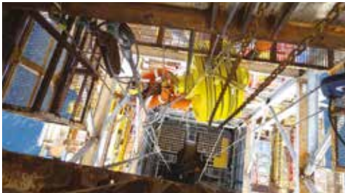
Rig builders with rope access skills assist the removal of the crown sheaves, 150ft up the Thistle derrick as part of the drilling maintenance programme.
