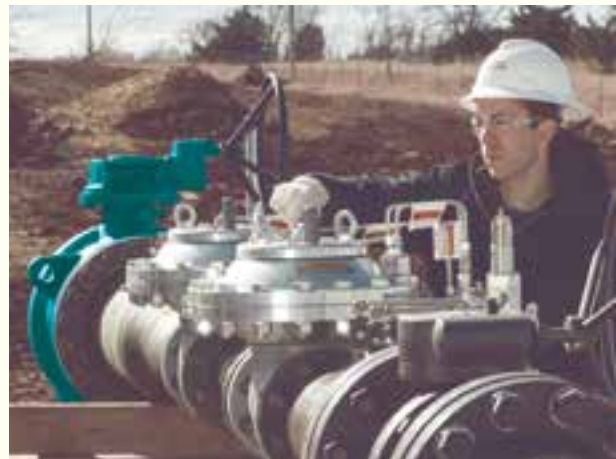
Oklahoma Natural Gas completed a pipeline project to supply the Stillwater Energy Center with efficient natural gas.
