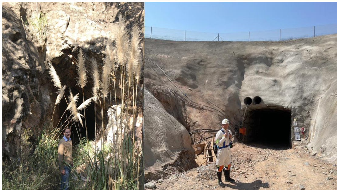
IMAGE 13: CEO JAC VAN HEERDEN AT THE QALA SHALLOWS BOX CUT BEFORE (LEFT) AND AFTER (RIGHT) REFURBISHMENT
