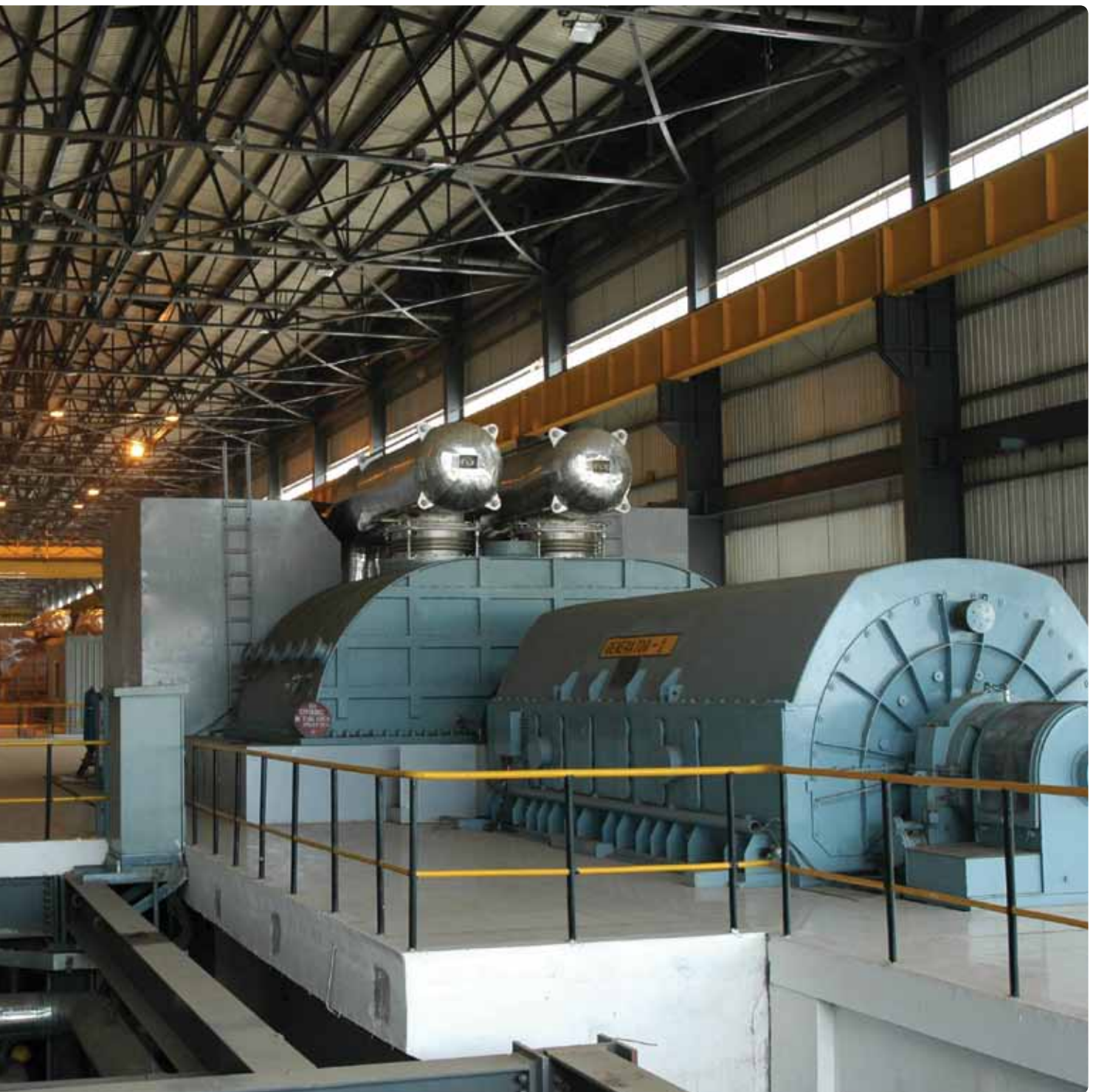
Above: Turbine Generator of the 1,215MW Power Plant, Jharsuguda.
