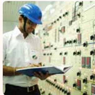
Above: Engineer verifying operating parameters at electrical control room of switchyard, BALCO.
