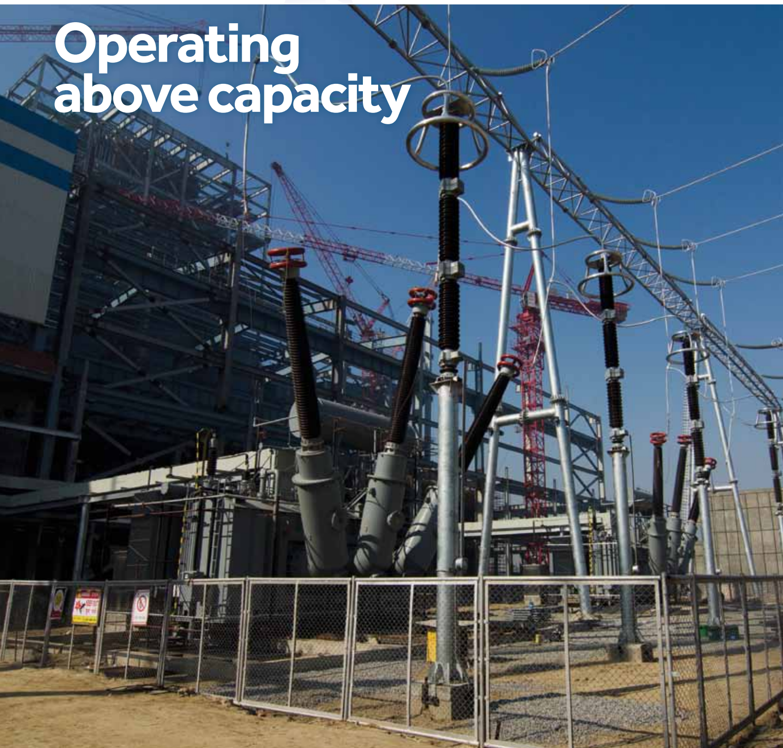
Above: Switchyard, Talwandi Sabo project.
