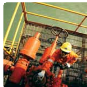
Above: Ravva offshore terminal, Cairn India.
