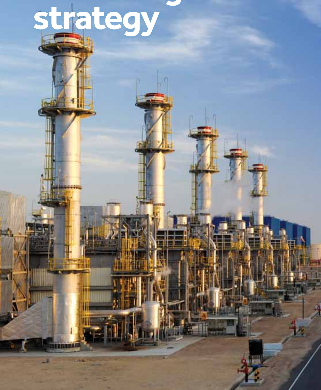
Above: Mangala processing terminal, Cairn India.
