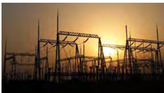
Caption: Switchyard, 2,400MW Jharsuguda Power Plant.
