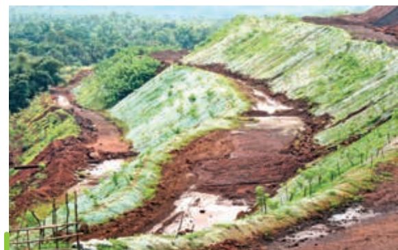
Below: Geotextile laid on dump slopes for dump stabilisation at Codli mine
