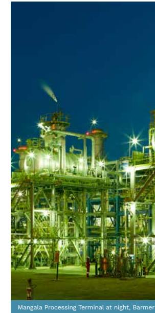
Mangala Processing Terminal at night, Barmer
