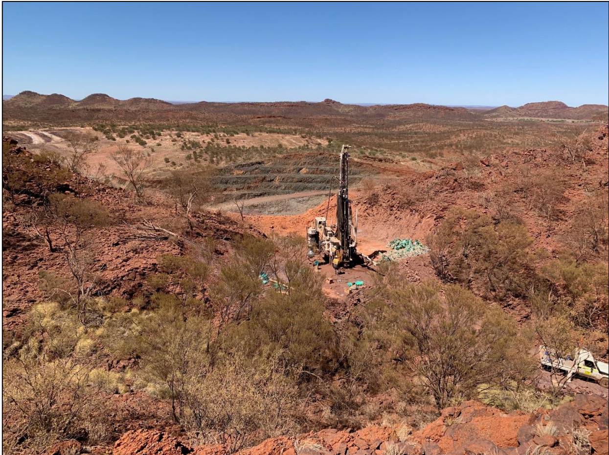
Figure 8: RC drilling for down plunge extensions at the Waugh Pit completed in December 2020
