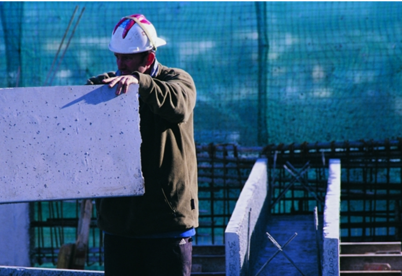
Stresscrete's timely production and delivery of pre-cast products was a crucial factor in meeting the challenging construction timetable – one floor per week – for the PricewaterhouseCoopers Tower project, in Auckland.
