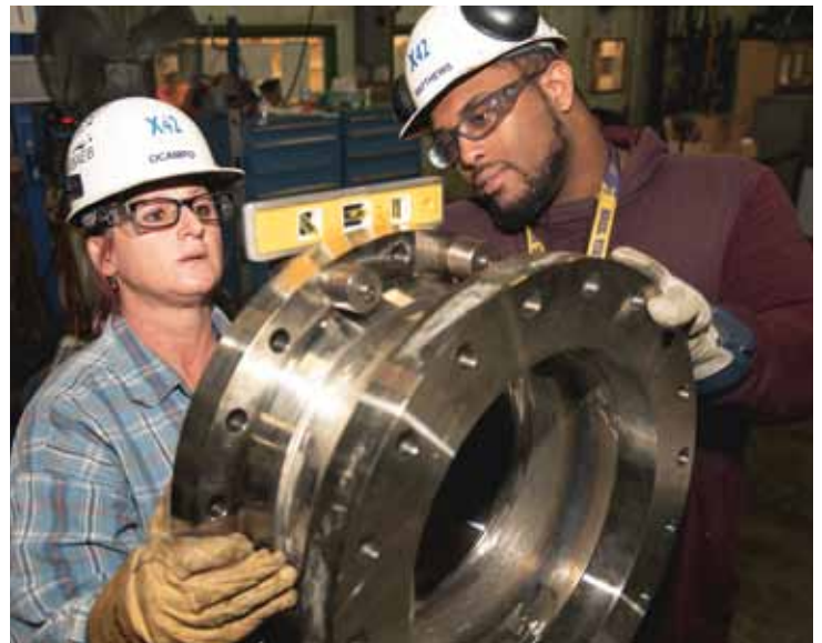
Newport News Shipbuilding employees (L-R) Tonja Ocampo and Davin Matthews align and level a pipe flange before tack welding in place.
