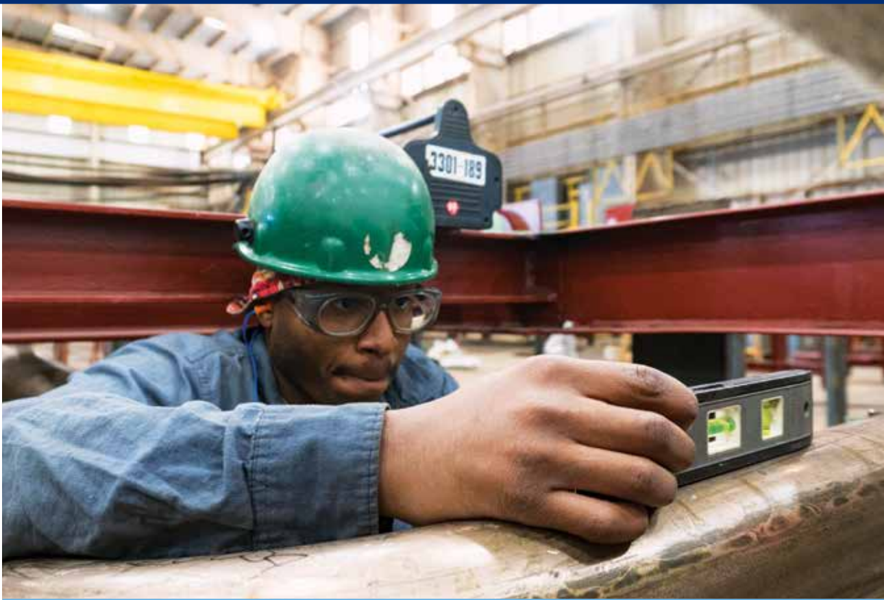
Ingalls Shipbuilding employee Jovan Joseph works on amphibious transport dock Harrisburg (LPD 30). Harrisburg will be the 14th San Antonio -class LPD delivered by Ingalls.
