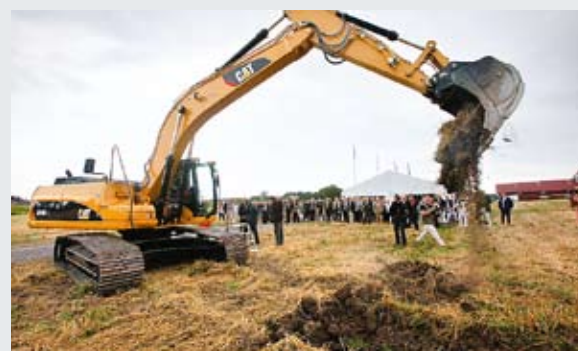
The ground-breaking ceremony for the new sawmill next to Braviken Paper Mill on 11 August attracted a great deal of media attention and invited guests.
