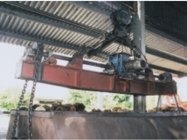
Renold PM40 gearbox installed in a palm oil mill in Malaysia.
