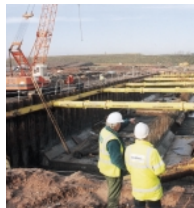
Renold Hydraulics & Variators, Bradford, produced this very large hydraulic excavation support system for work at Birmingham International Airport.
