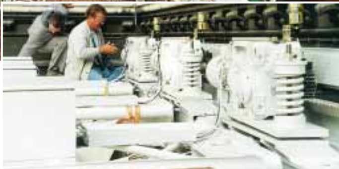
Renold Powermaster gear units are used to open and close the roof structure over the courtyard of the City Hall in Vienna.
