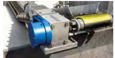
Tension release backstop in a conveyor.
