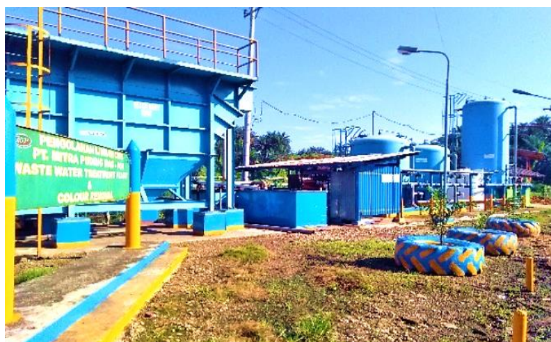
Waste water treatment plant
