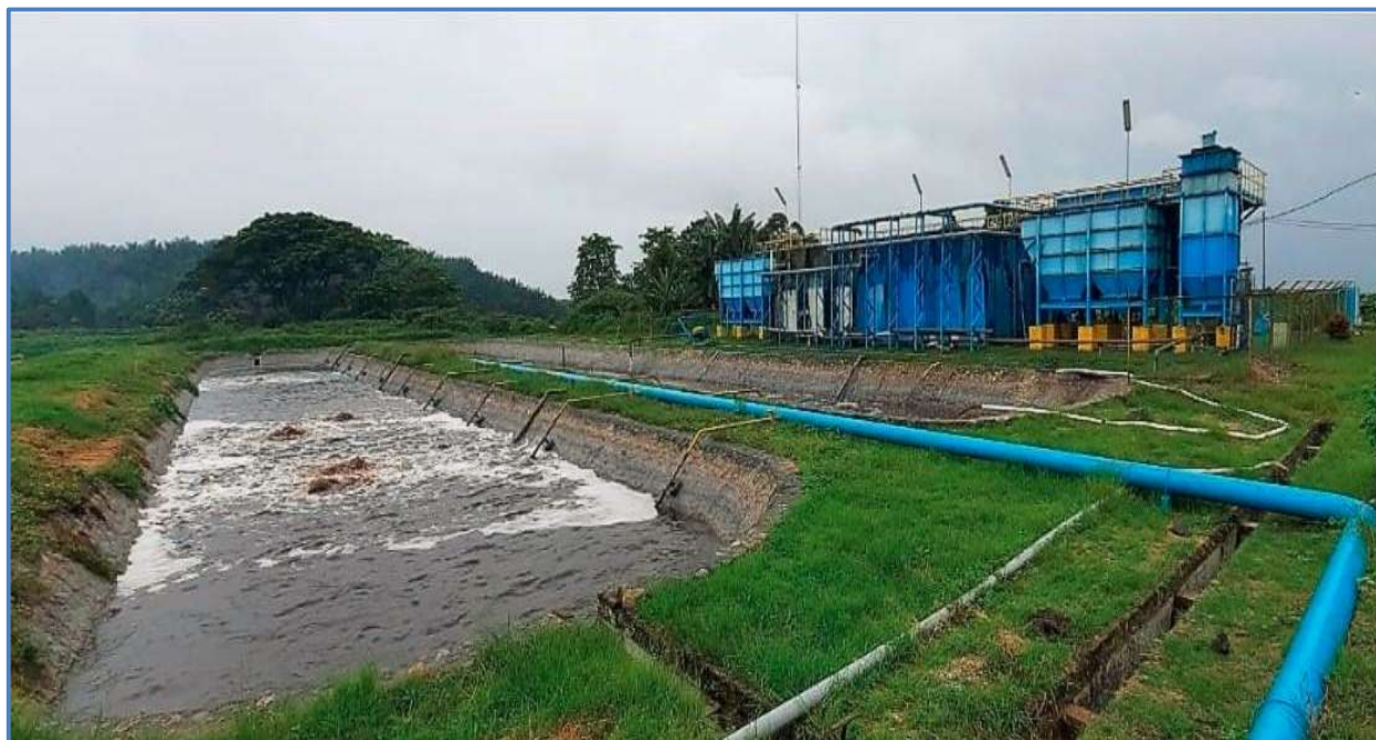
Aeration ponds and tanks for treatment of mill effluents
