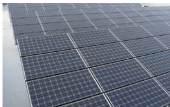
Solar power generation equipment at Group's main computer center
