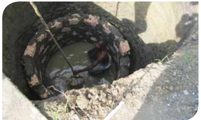
The water table is found and the inside wall of the well is constructed using stones and cement
