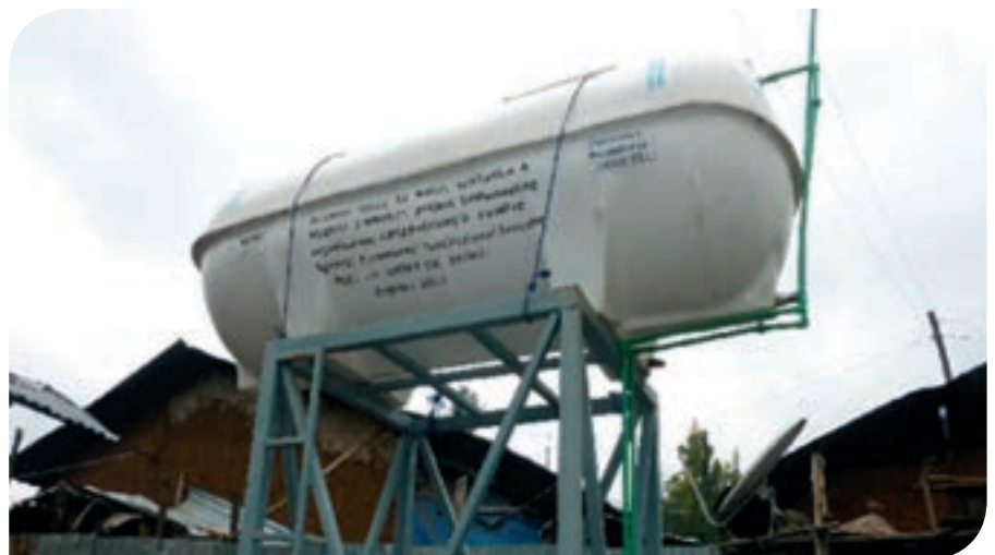
Kechene new water and sanitation facilities.
