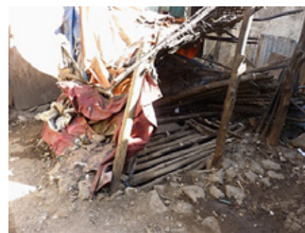
Condemned water facilities
