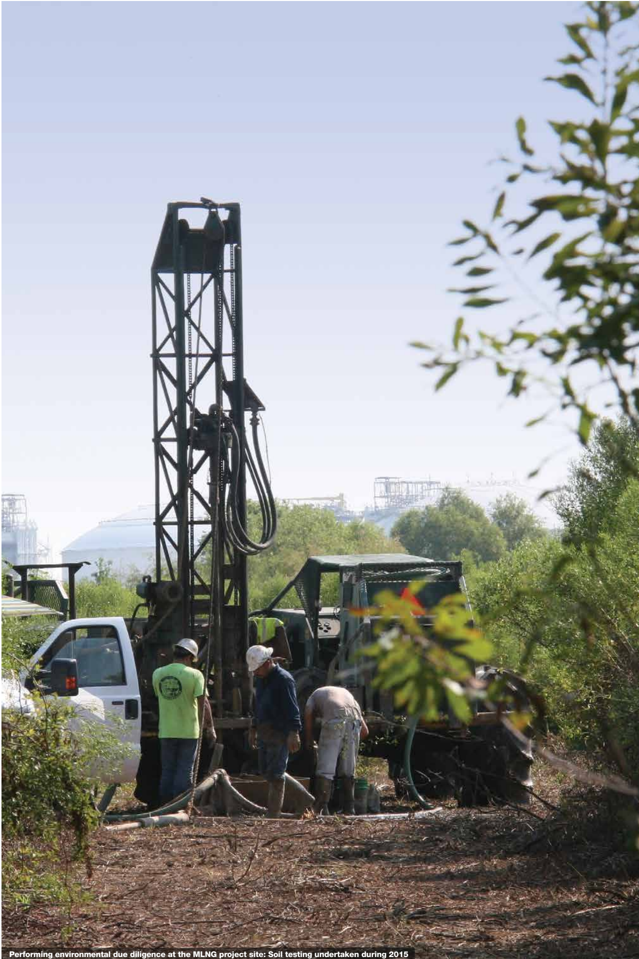
Performing environmental due diligence at the MLNG project site: Soil testing undertaken during 2015
