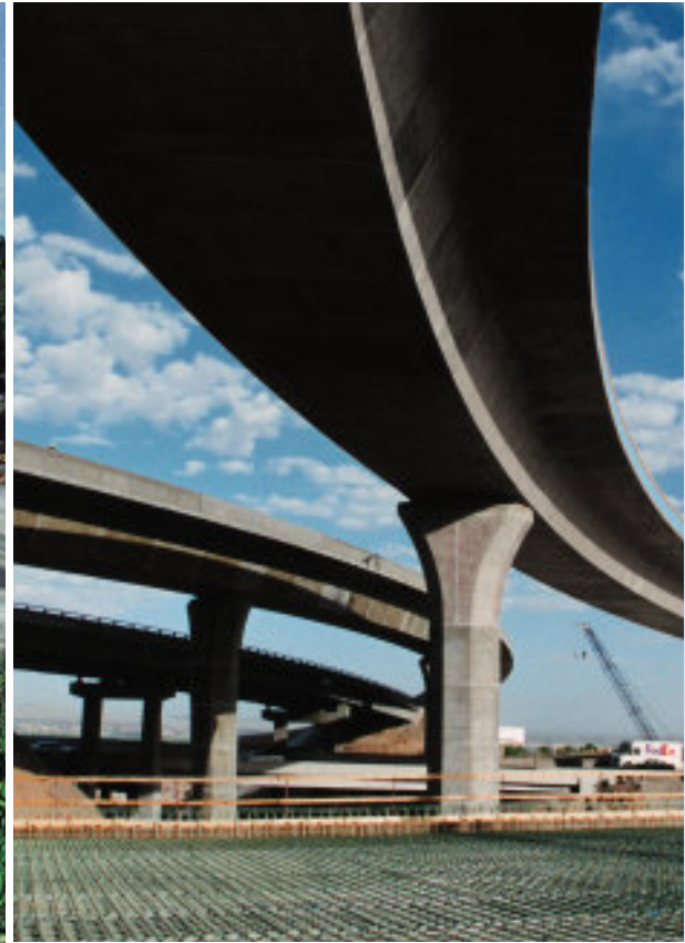
Waycor, in the Western region, was the sole supplier of construction materials on the rebuilding of the "Big-I" in Albuquerque, New Mexico. This is the largest single highway project ever awarded in New Mexico and will cost US$270 million, using 127,000 cubic metres of concrete and 900,000 tonnes of aggregates.
