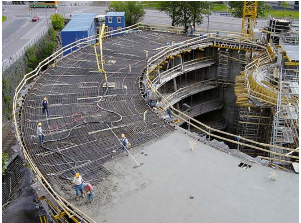
Concrete being pumped into a floor in the extension to the Finnish Parliament in Helsinki. Lohja Rudus delivered over 10,000 m 3 of concrete to the architecturally innovative project.
