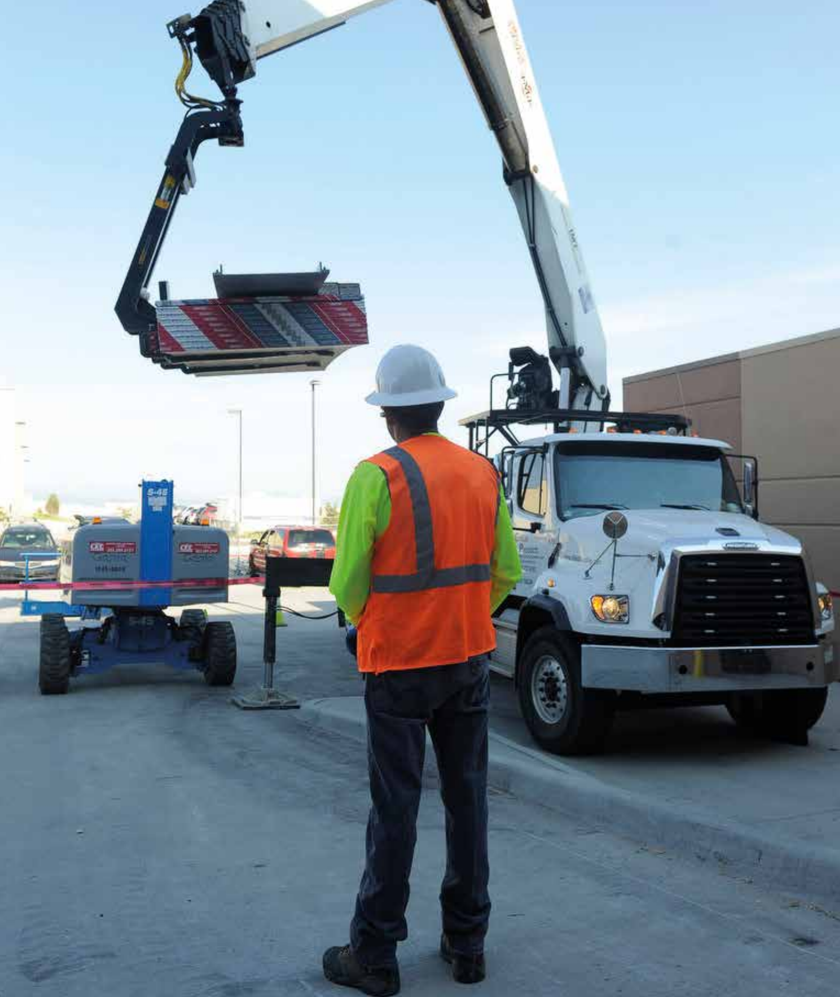
Truck Loader at Gypsum Products, Inc. a division of Allied Building Products, delivering 5/8" (13 cm) drywall to a commercial project in Denver, Colorado.
