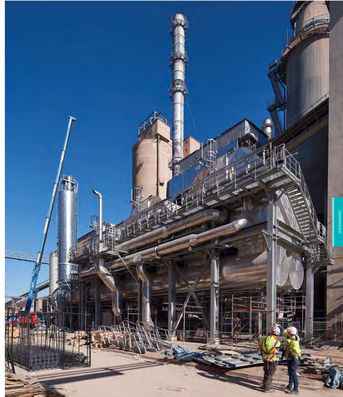
In July 2019, OPTERRA, part of CRH's Europe Materials Division and one of the leading cement producers in Germany, officially inaugurated a new exhaust gas purification system at its Karsdorf cement plant near Leipzig. The new filter technology, which includes a state-of-the-art AUTONOX ® Low Dust System installed on the existing kilns, enables the factory to comply with new limits for dust, ammonia and nitrogen oxide emissions.
