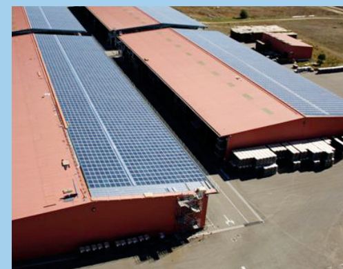
O-I's Bezier, France, plant – already an O-I sustainability leader – will play a role in the larger green energy movement. In 2010, solar panels were installed on the roofs of the plant's warehouses. O-I expects the panels, which cover four buildings and a total surface area of 10,000 square meters, to produce 1.7 gigawatt-hours of electricity annually for area businesses – enough energy to power a 2,300-resident community for a full year.
