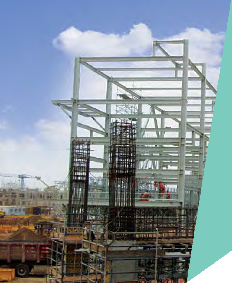
Petrochemical complex in Mexico: 10,000 workers employed for the construction work and 58% from the installed project
