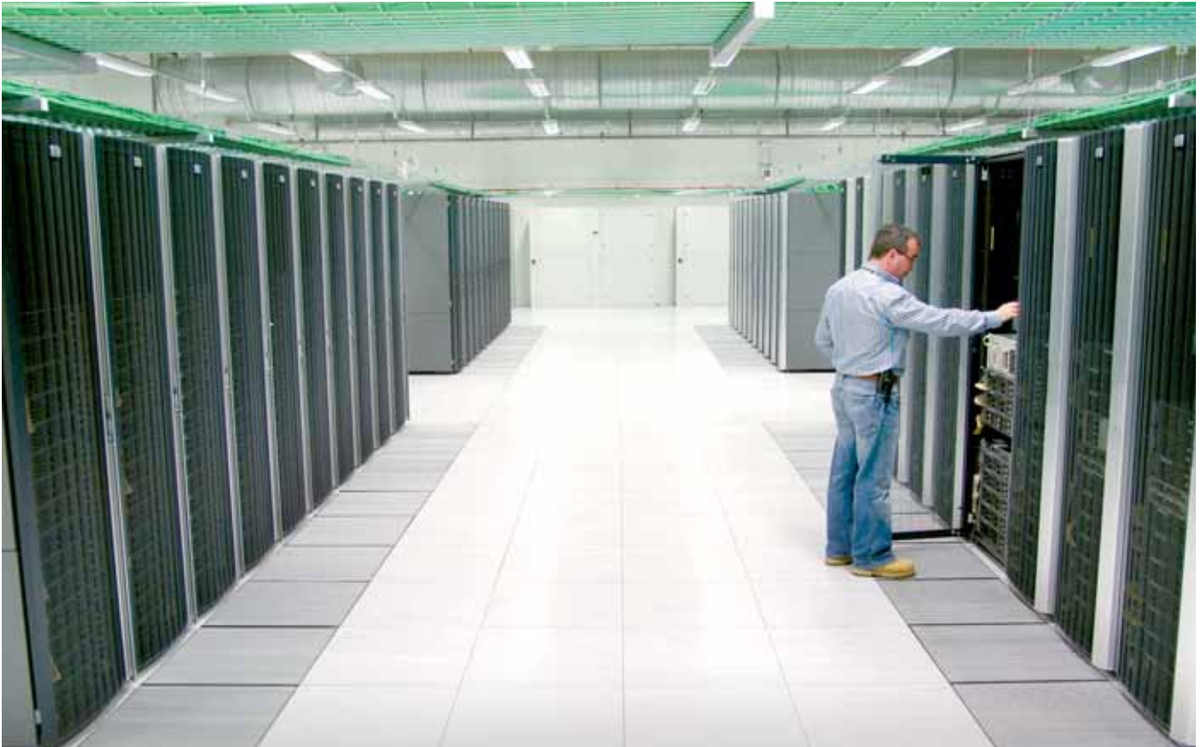
Leveraging its expertise in delivering 100% availability specialised data centre management, Citadel100 delivers a range of customised solutions ranging from co-location suites to dedicated data vaults.
