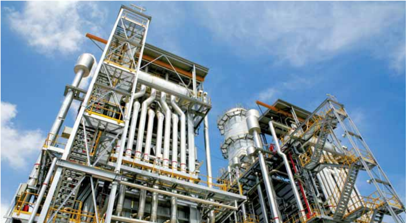
The Keppel Merlimau Co-generation Power Plant has been contributing to earnings since operations in 1H 2007.
