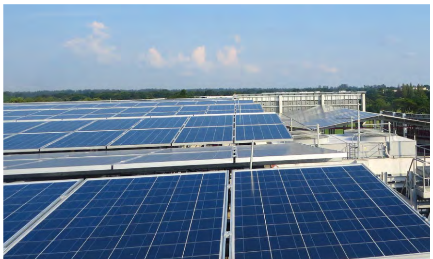
Keppel Land's corporate office at Bugis Junction Towers is fully powered by solar energy from Keppel Electric.
