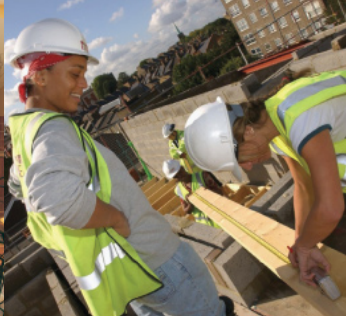
Above: As part of the company's efforts to encourage more women into construction careers, Lovell has been providing 13 week placements for trainee carpenters and plumbers at two of its London housing sites through the Building Work for Women Partnership.
