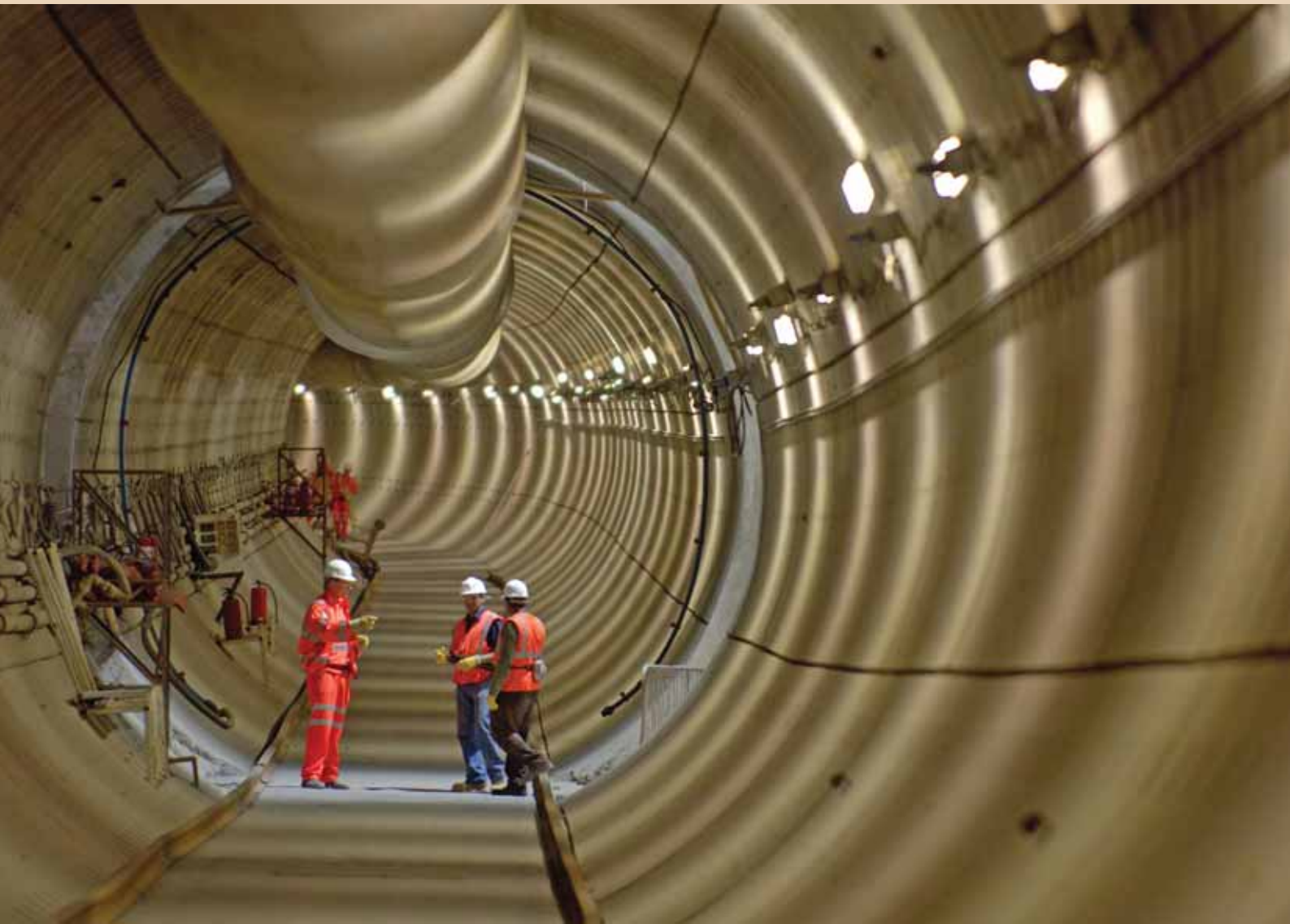
Above: Morgan Est's £90m programme of tunnelling projects for BAA at Heathrow's new Terminal 5 reached the final stage with the Piccadilly Line and Heathrow Express extensions nearing completion.
