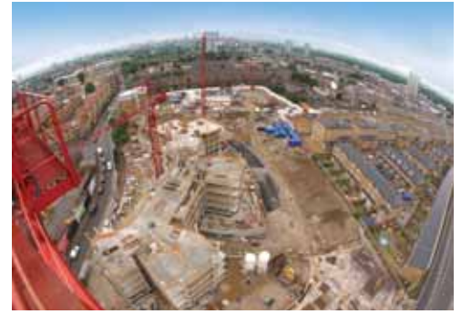
Top: Heart of Bow: A bird's-eye view of Lovell's £54m mixed tenure development in London's East End. The 279 houses and flats for affordable rent, shared ownership and open market sale are being built near the site of the 2012 Olympic stadium.
