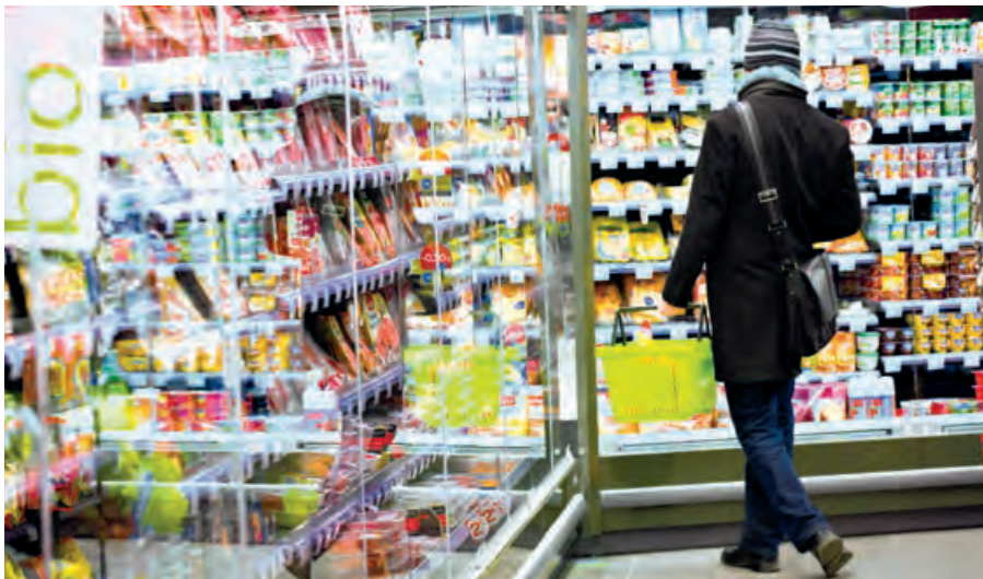
01 Closed refrigeration units is one of the Group's initiatives for reducing energy consumption in its stores. Manhattan Express store in Brussels (Belgium).
