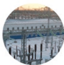
The 330 kV Electric Energy Ring in St. Petersburg
