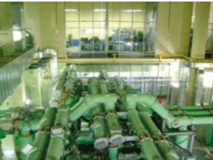
Switchgears for the secondary distribution systems in the Skolkovo substation
