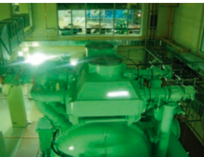
Gas insulated transformer in the Skolkovo substation
