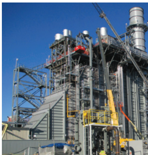
Our Garrison Energy Center, a 309 MW combined-cycle power plant, is scheduled to commence commercial operation in Delaware in 2015.
