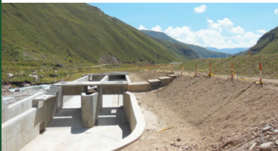
Photograph: Gravel trap, Canchayllo, Peru.
