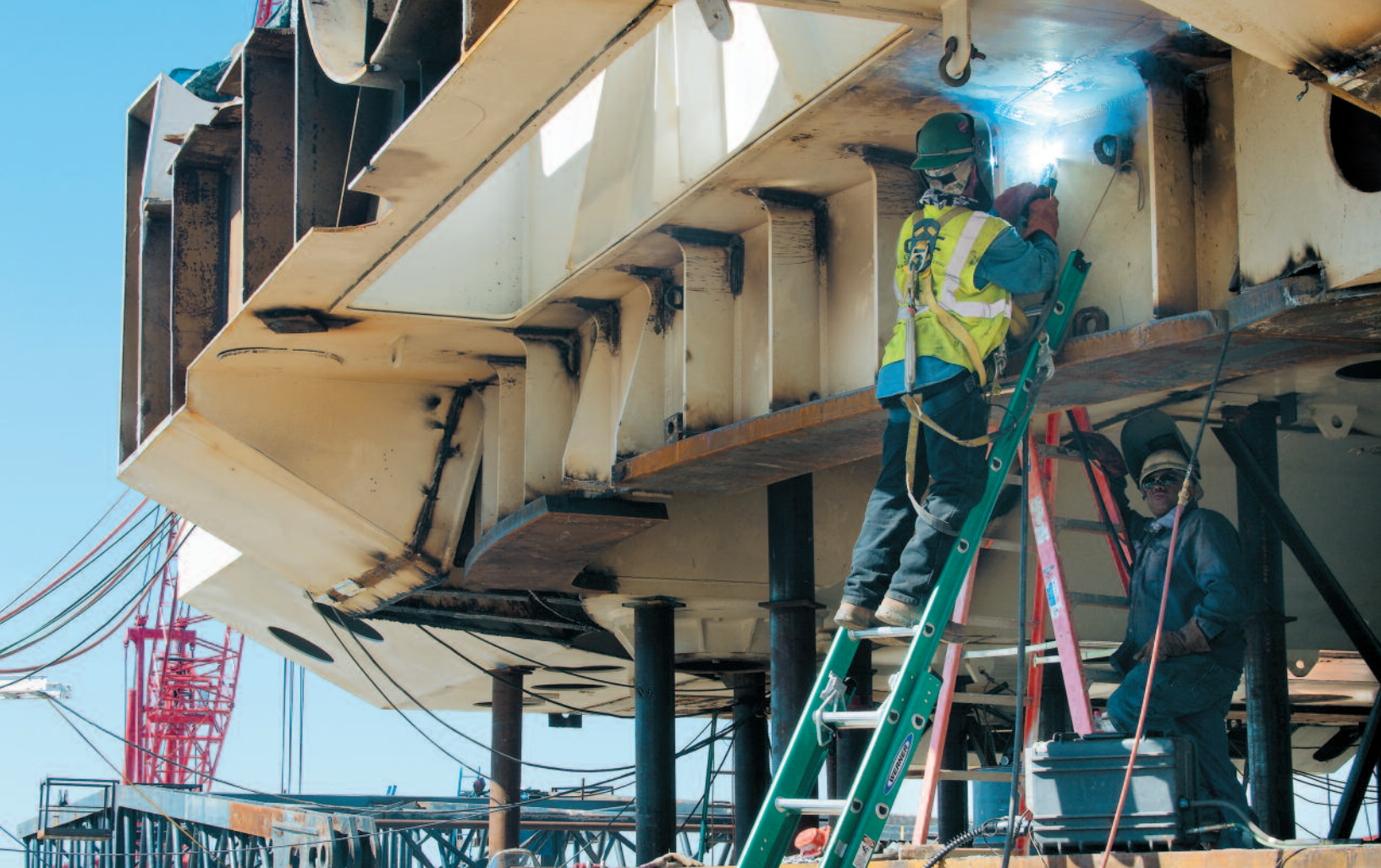
Much of the development work at the new Liberty Mine in Mississippi involves assembling mining equipment, such as this dragline that will eventually be used to remove overburden.
