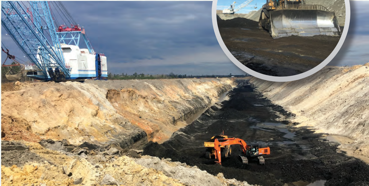
Our skilled mining experts provide comprehensive mining services, including permitting, mine planning, excavation, load and haul and reclamation. Shown are mines in Texas and North Dakota (right).
