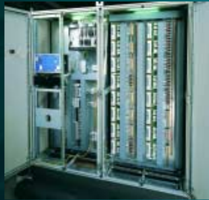
Integrated digital control system
