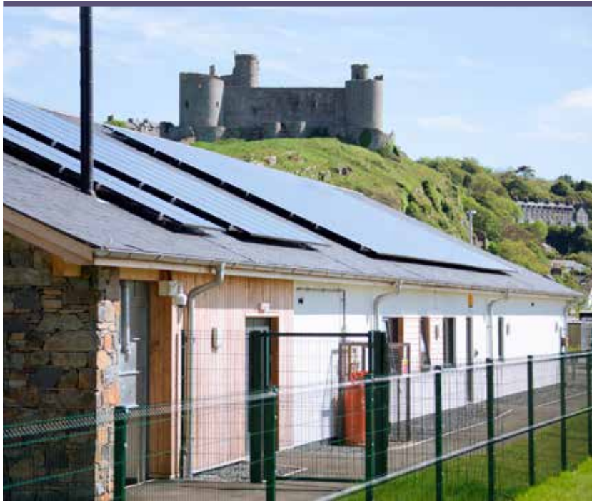
Photovoltaic cells at Arudwy Health Centre, Harlech
