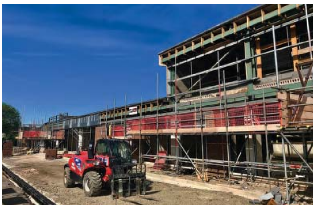
New development at Baddeley Court, Newport, Shropshire. Opposite page: artist's impression of the finished project, above and left: in progress May 2019.
