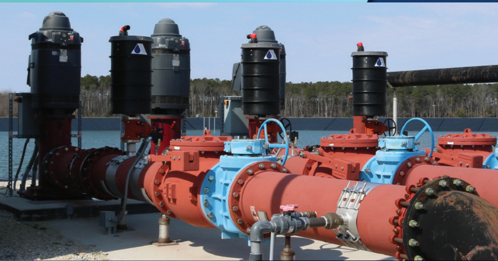
The effluent from Artesian's lagoon systems is treated to land application standards for spray irrigation, while retaining its high-nutrient content.
